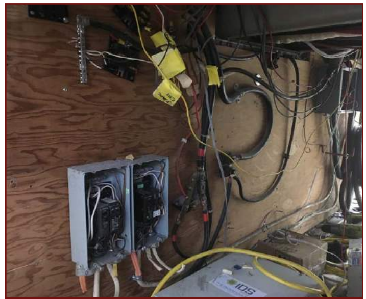
The electrical panel before renovations.
