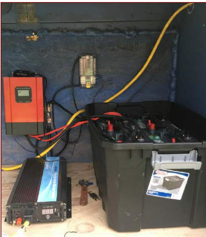
A look inside the electrical bay.
