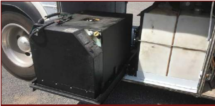
Onan 7500W generator.
