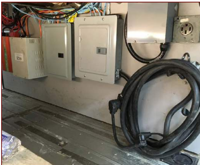
The electrical panel now (Pictured from the left side of the bus).
