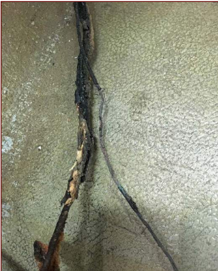
These were wires that had current flowing through them behind the walls. Pretty scary!
