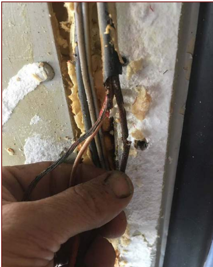
These bare wires were also behind the walls and had current flowing through them.
