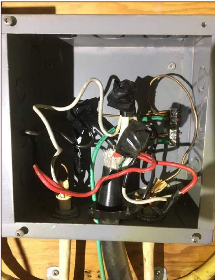
This was what we found inside the electrical boxes. Not reassuring.
