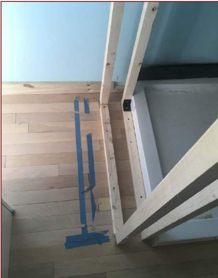
We taped out our layout but gained and lost inches when actually building.
